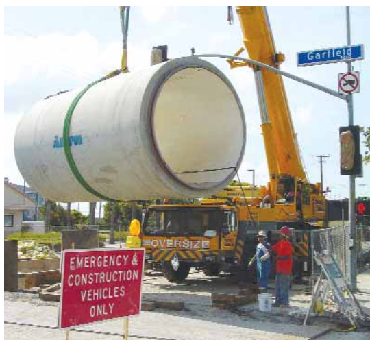
USING A HYDRAULIC CRANE TO LAY 108-INCH PIPE ON THE SOUTH SIDE OF THE GARFIELD INTERSECTION OF BUSHARD.
