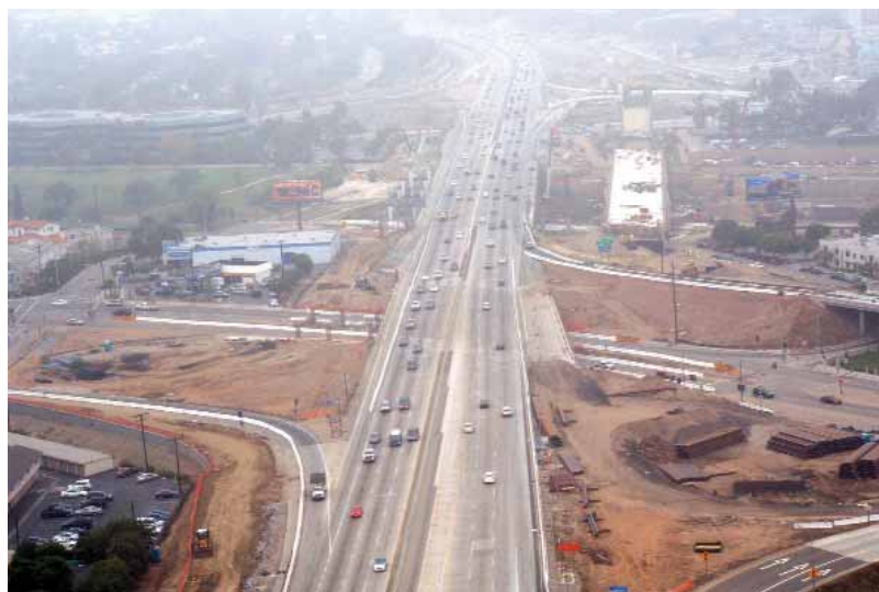
A section of GMR SR-22 at the beginning of work (top) and the finished product (bottom).
